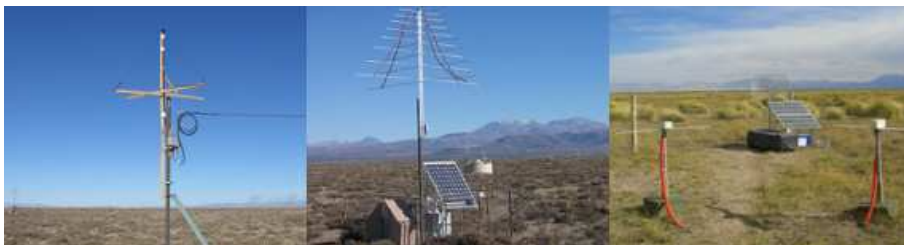
Figure 3.6: Different antenna prototypes, installed near Malargüe [29].
