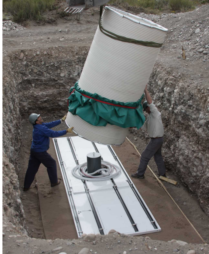
Figure 4.7: Deployment of the 5 m 2 prototype at the SD station Corrientes in November 2009 [45]; in order to retain access to the electronics installed in the center of the module (inside the grey casing), the prototype is equipped with a manhole (white tube).
