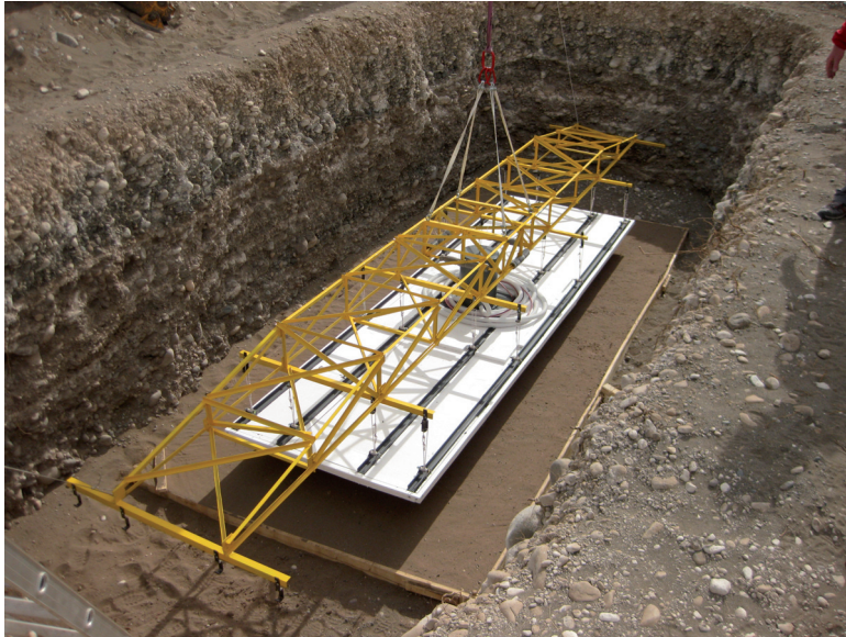
Figure 4.5: During the installation of the first 5 m 2 MD module at Corrientes . The yellow scaffold holds the detector in a horizontal position. It is also suited for the 10 m 2 modules. The dome, which encloses the readout electronics and the PMT, and the u-profiles, that give stabilisation to the module can be seen. Styrene is attached to the module to protect it from the topside. A sand bed of \approx 20 cm height was prepared for the module to protect it from rocks in the soil below and to ensure a horizontal position. Except for the access tube, which enables maintenance of the PMT and the electronics, the pit was completely filled with soil as the last step of the mechanical deployment; image: November 2009.
